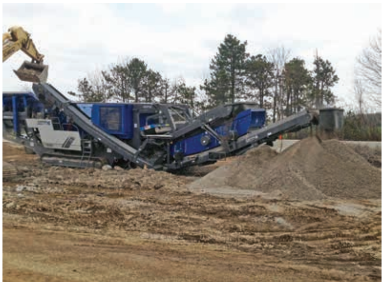
Shelly & Sands' Mobirex MR 110 Z EVO mobile impact crusher in I-71 median crushes existing concrete pavement
